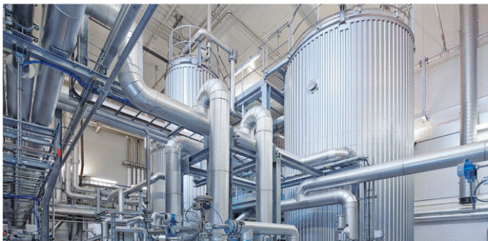
The biofuel is produced in this plant and used by refuse collection vehicles (RCVs)
